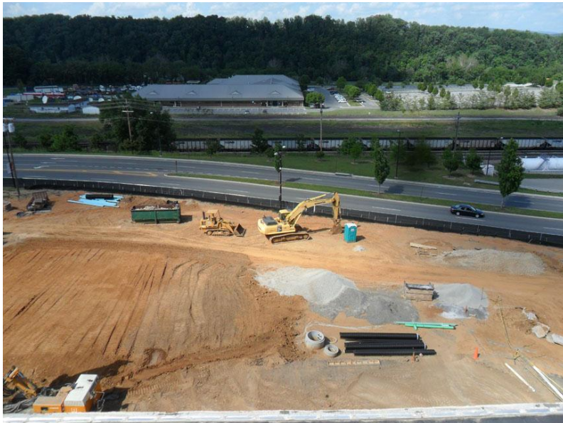
Image taken from the roof of Curie Hall, looking where the Curie parking lot used to be. The new planetarium will be near the light-blue plastic towards the left of the picture.
