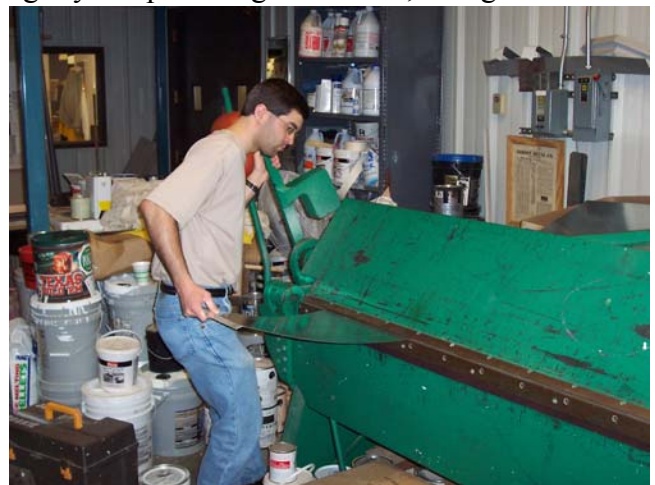
Using the sheet metal breaker to construct panels for the exit diffuser.
